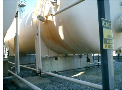
Additional Anchorage Required
