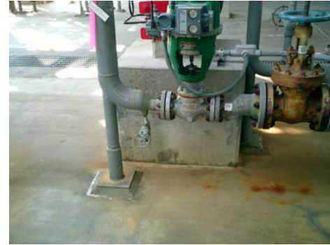
Piping Remediation Issue – Seismic Interaction
