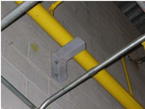
Piping Remediation Issue – Loss of Support
