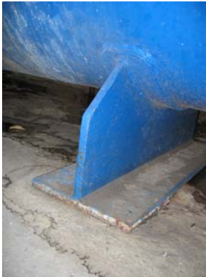
No Anchorage Identified During Walkdown
