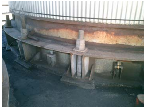
Additional Anchorage Required
