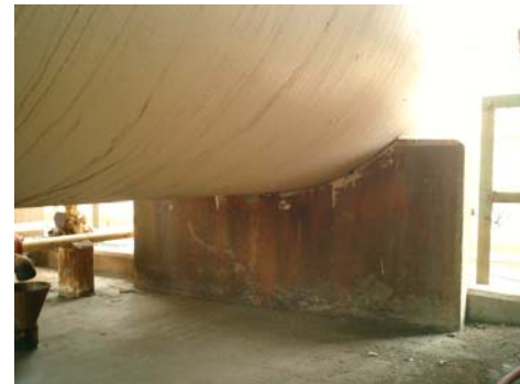
No Anchorage Identified During Walkdown
