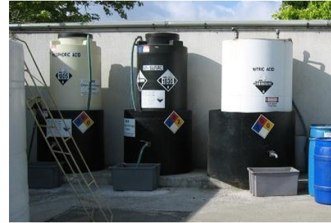
No Anchorage Identified During Walkdown
