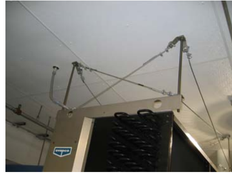
Good Equipment Bracing
