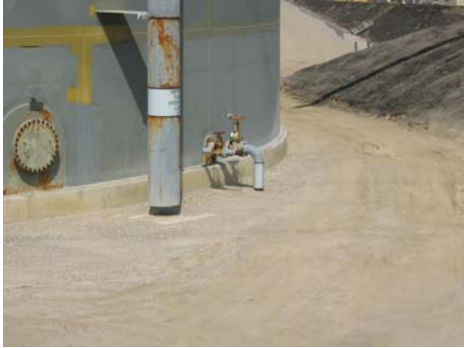
Piping Remediation Issue - Flexibility
